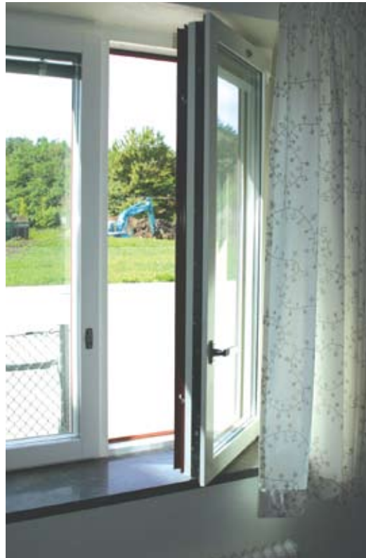
Security system window-contacts are co-utilized by the climate system
