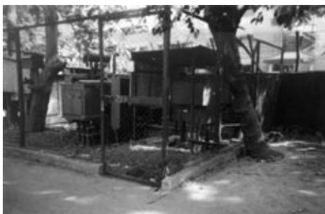
Fig. B39 : Outdoor substations without enclosures
